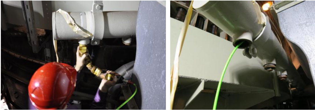
Figure 11: Left, inserting the snake into the nitrogen line. Right, a view down the nitrogen line during the inspection.
