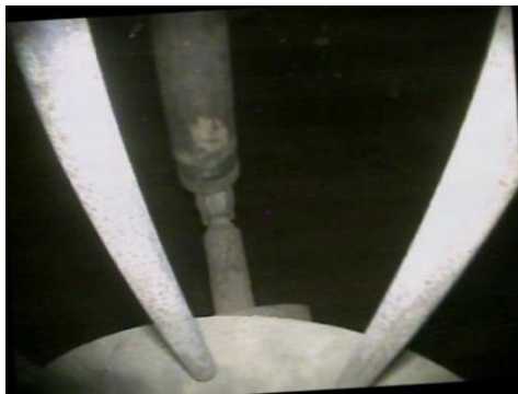
Figure 7: An image of the inside of the moisture separator. The robot is suspending itself from the pipe entering at the top of the vessel
