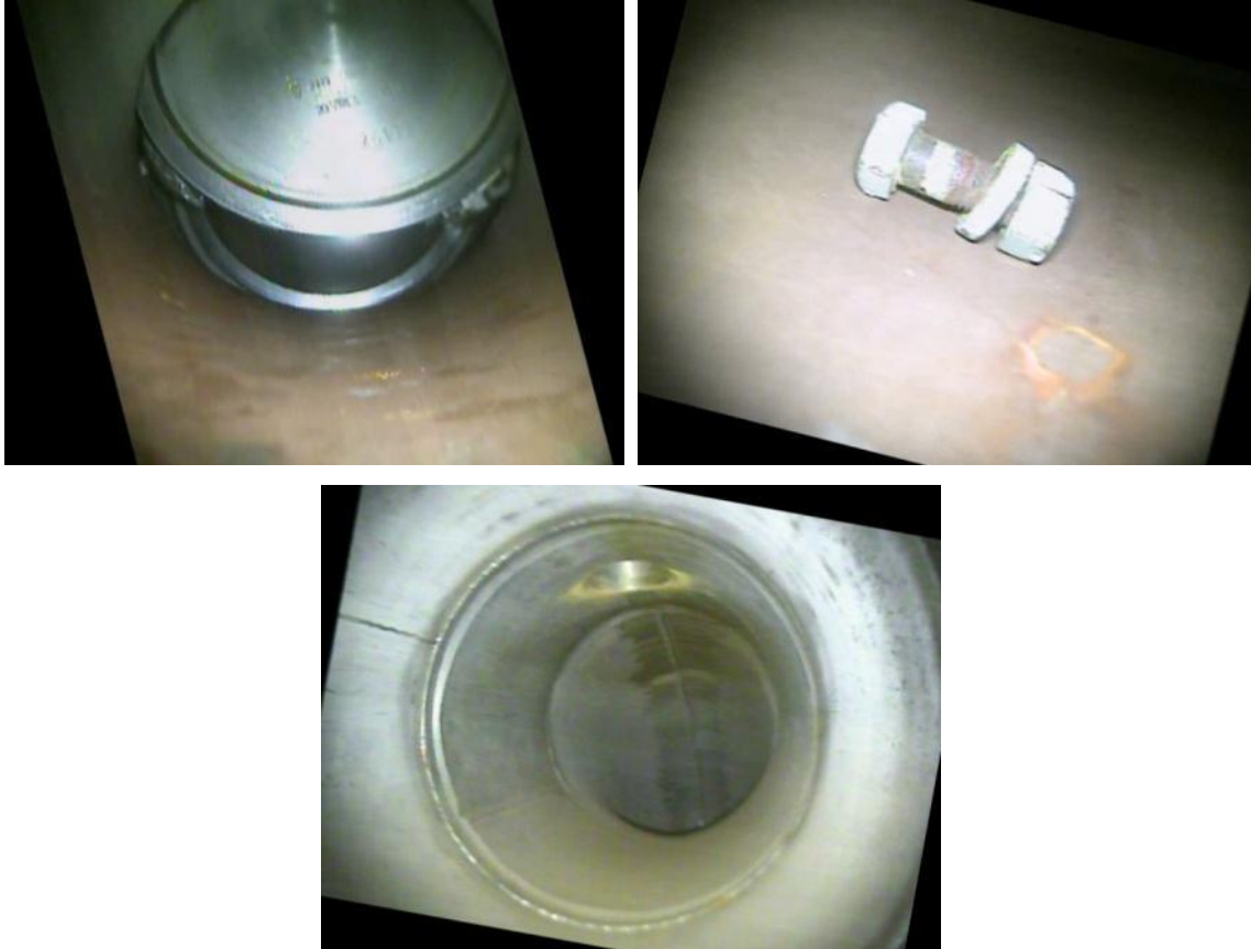
Figure 11: Views from inside the steam pipe in the upper reactor area. Top left, a partially open valve. Top right, a nut and bolt. Bottom, a 90-deg bend in the pipe with a smaller pipe junction.
