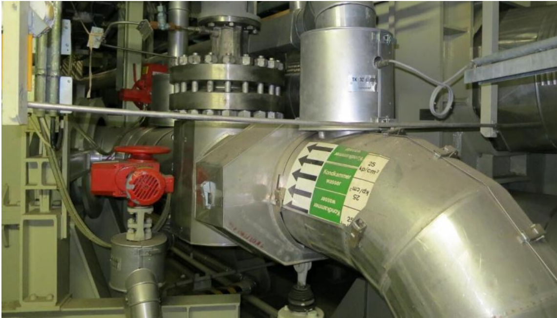
Figure 10: External view of the valve and steam piping that the robot traversed.
